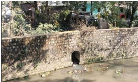
Image 7-9: Greywater discharge into Rambha River near Barrage Colony
